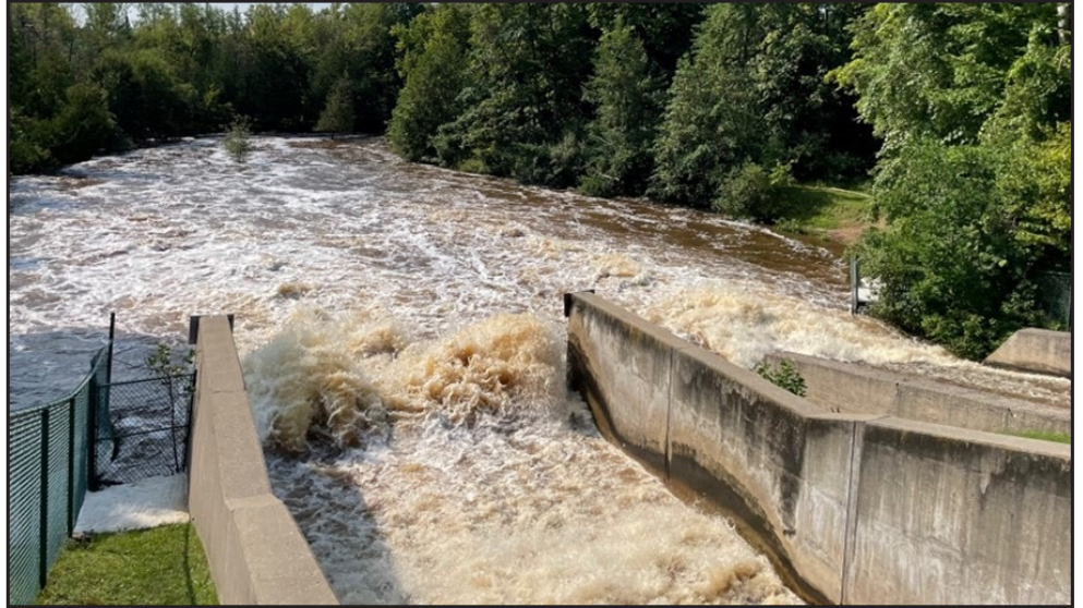
Spillway of the Bellaire Dam a day after a heavy rain event
